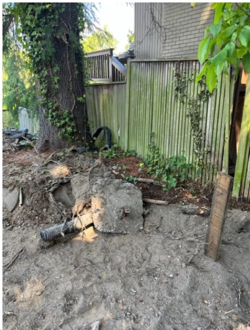
Wood marker to right of photo indicates 5' deep excavation, about 10' from tree.
